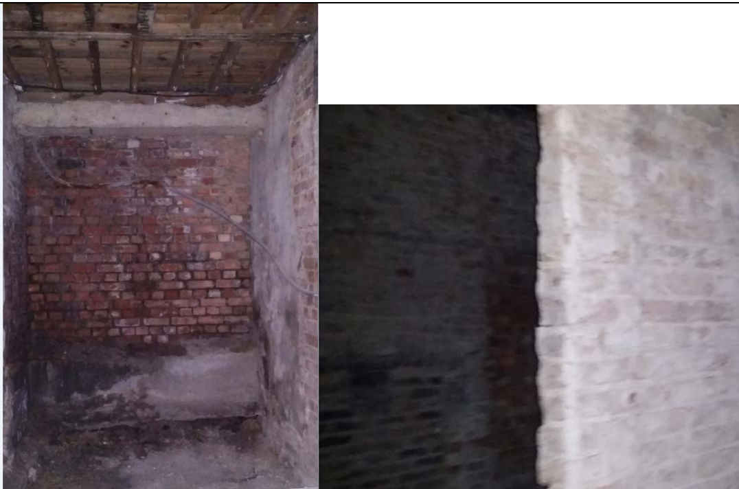
Basement of 32 Blomfield Villas (indicative of the size/state of all the basement spaces to be turned into 3 bedroom flats.)
