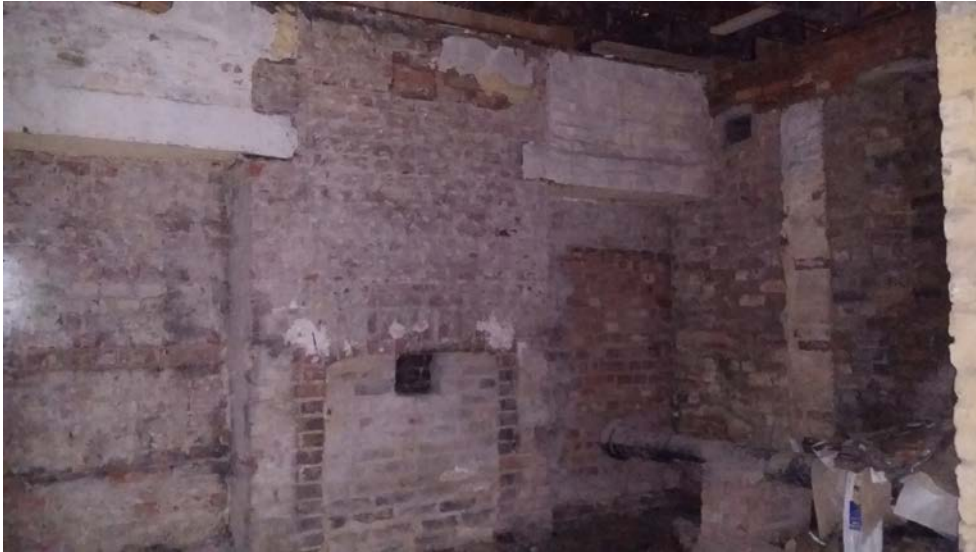
Basement of No.28 Blomfield Villas (indicative of the size/state of all the basement spaces to be turned into 3 bedroom flats).
