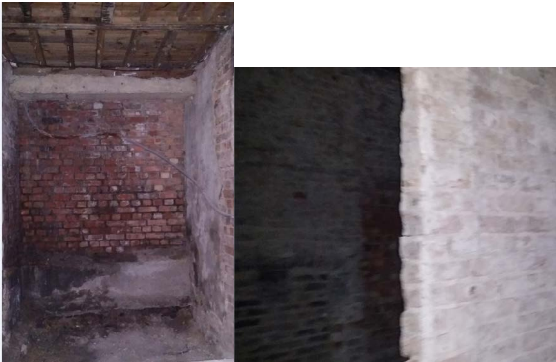
Basement of 32 Blomfield Villas (indicative of the size/state of all the basement spaces to be turned into 3 bedroom flats)
