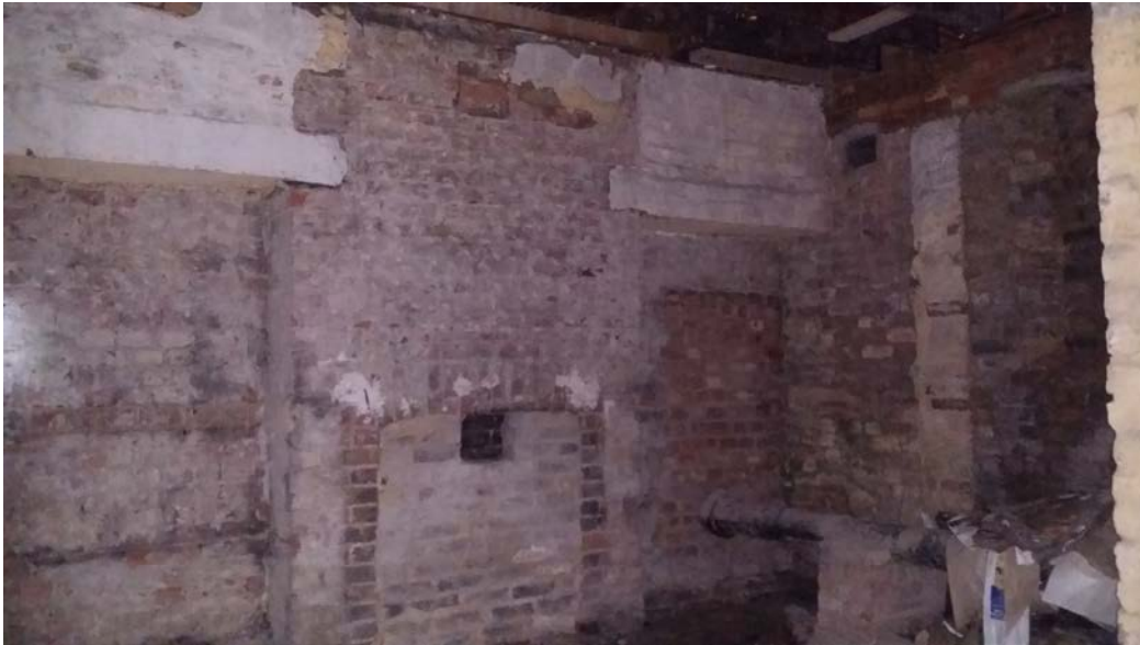
Basement of 28 Blomfield Villas (indicative of the size/state of all the basement spaces to be turned into 3 bedroom flats)
