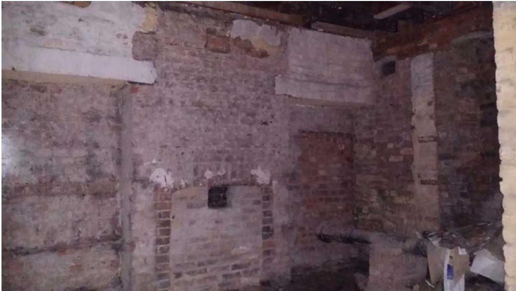
Basement of 28 Blomfield Villas (indicative of the size/state of all the basement spaces to be turned into 3 bedroom flats).
