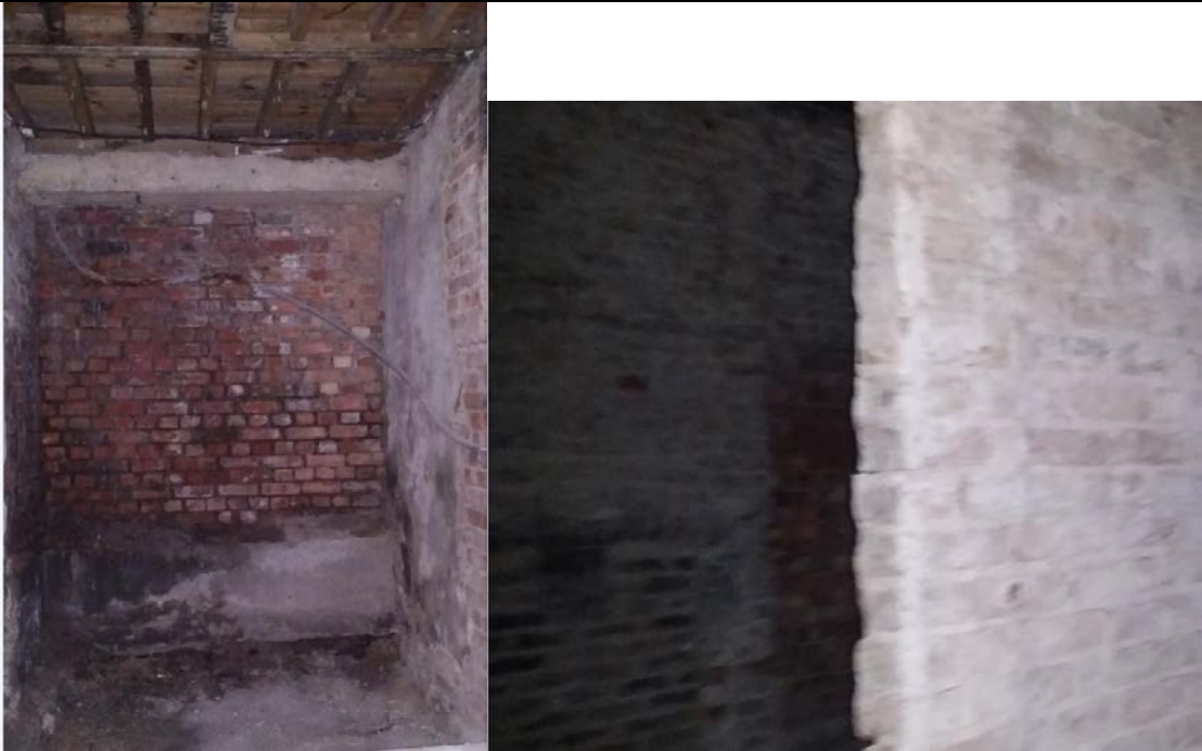
Basement of 32 Blomfield Villas (indicative of the size/state of all the basement spaces to be turned into 3 bedroom flats).
