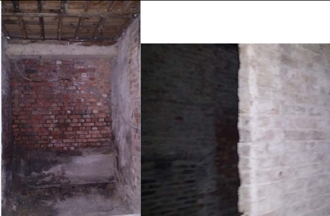
Basement of 32 Blomfield Villas (indicative of the size/state of all the basement spaces to be turned into 3 bedroom flats).
