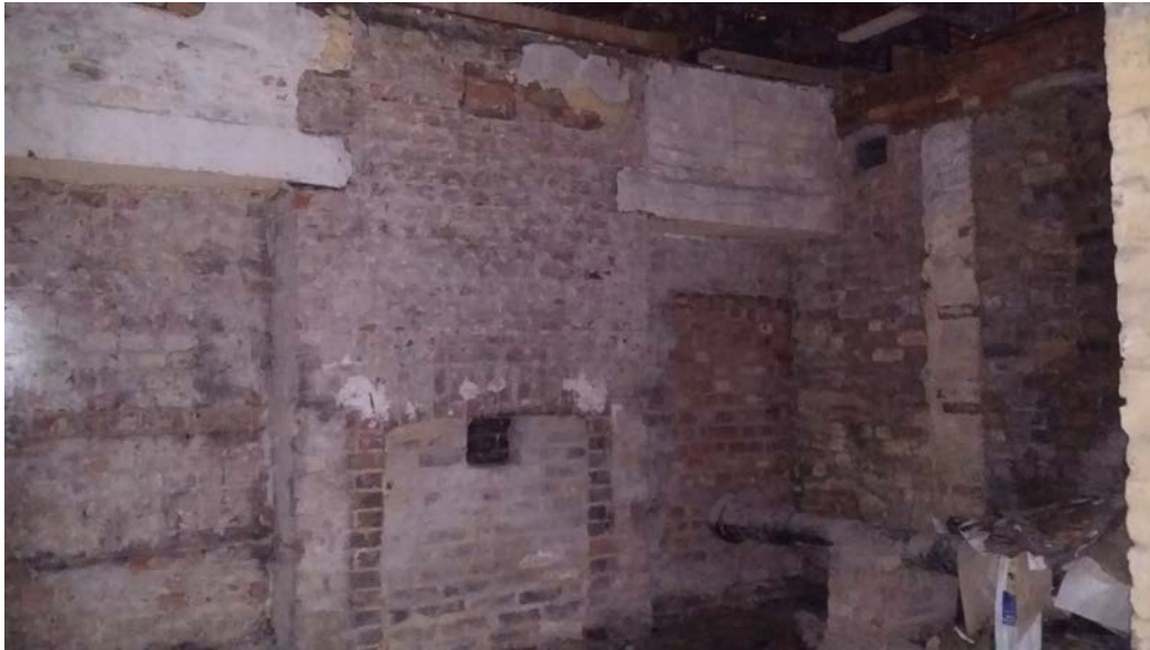
Basement of 28 Blomfield Villas (indicative of the size/state of all the basement spaces to be turned into 3 bedroom flats)
